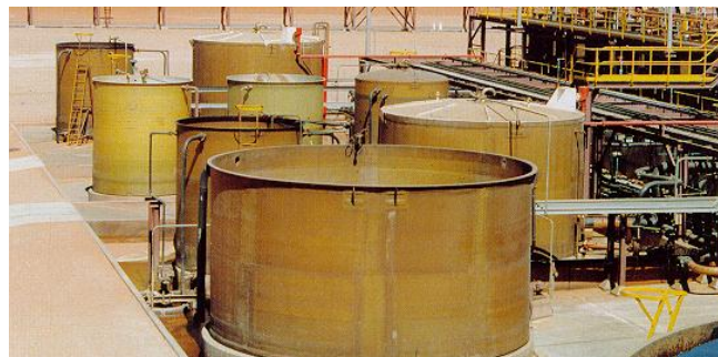
Figure 8. Reagent Storage Tanks
