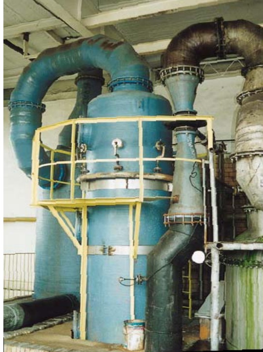
Figure 7. Acid Vapor Collection System
