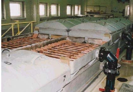
Figure 9. Electrowinning Cells for Copper Recovery
