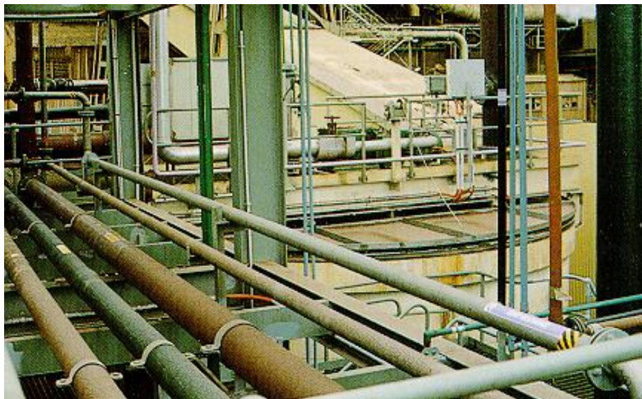
Figure 4. FRP Sulfuric Acid Piping
