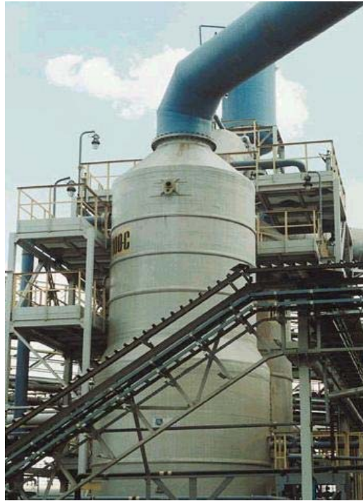
Figure 5. Sulfur Dioxide Absorption Tower
