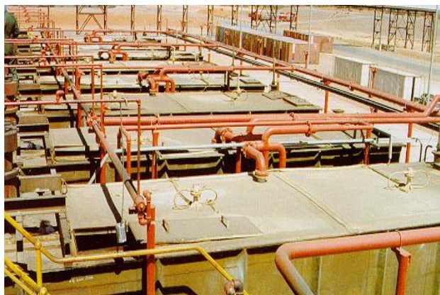
Figure 6. Solvent Extraction Mixer-Settler Tanks
