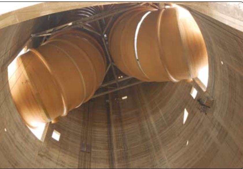
Fig. 3. FRP Stack liners.
