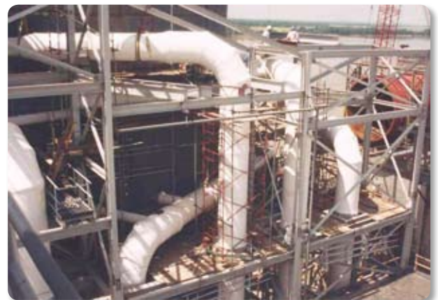
Fig. 4. FRP Abrasion resistant limestone slurry piping to power plant scrubber.
