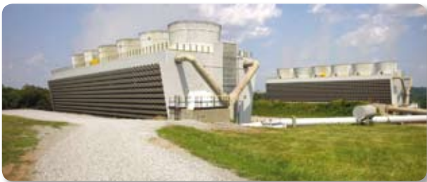
Fig. 6. Composite cooling towers at 750MW Midwest Power Plant designed for 50-plus years service life.
