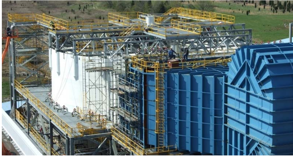
Figure 9. Scrubber and Ductwork in a 600MW Power Plant.
