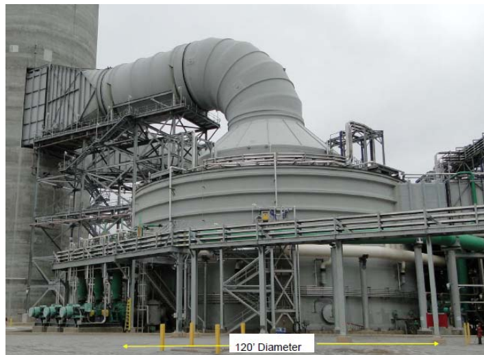
Figure 10. Scrubber and ductwork in a 950MW power plant.
