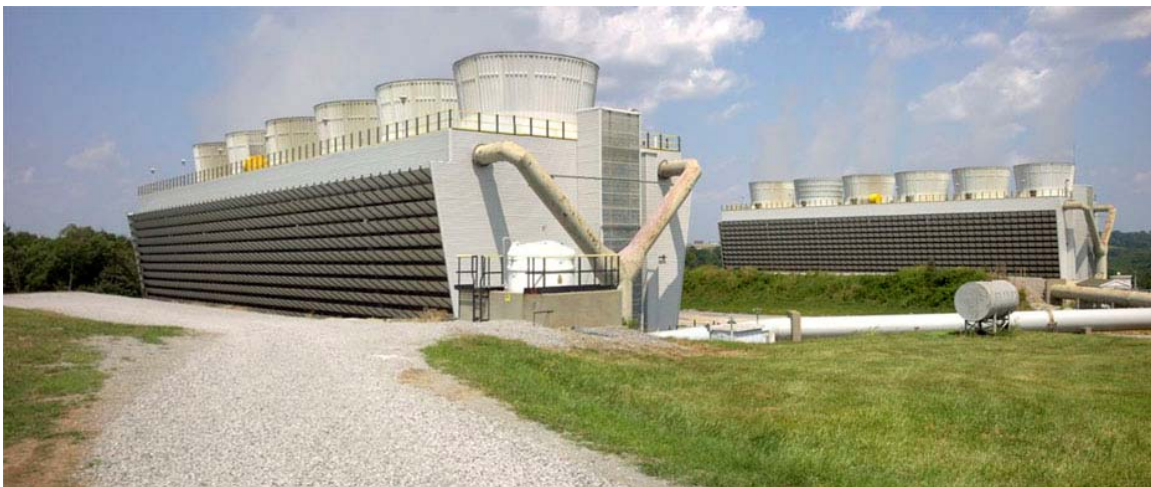
Figure 11. FRP Cooling Towers at 700 MW Midwest Power Plant.
