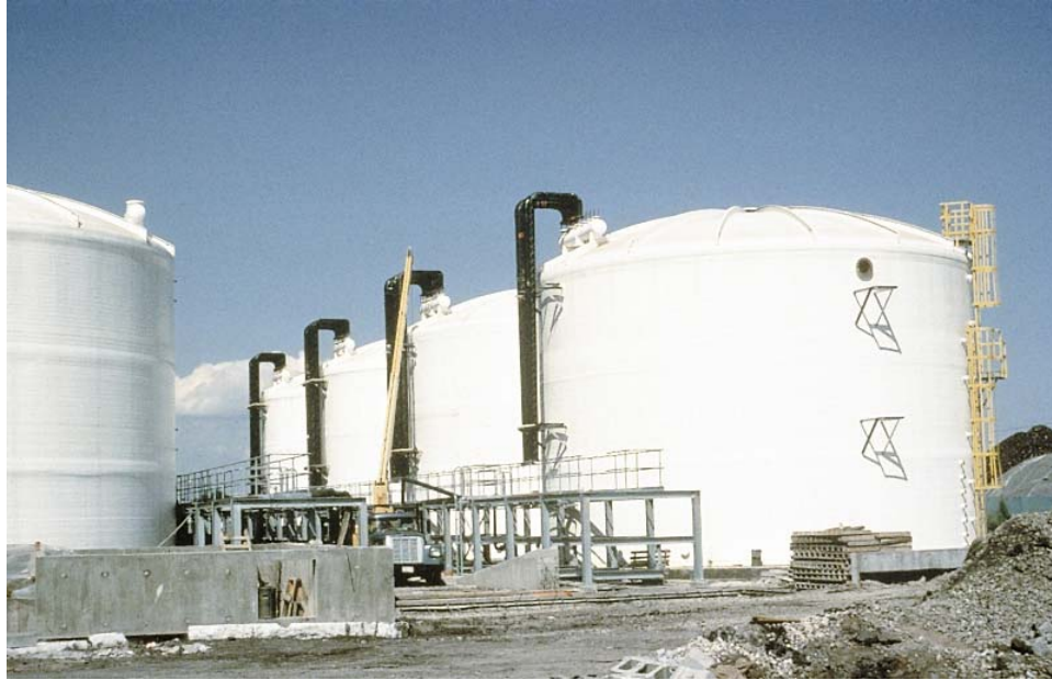
Figure 14. Large Field Wound Hot Water Storage Tanks
