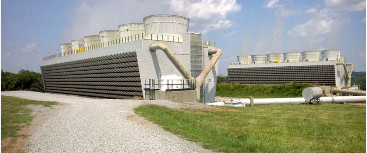
Figure 18. All FRP Cooling Towers
