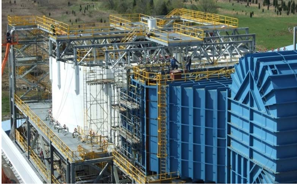
Figure 16. Large Flue Gas Scrubber for a Power Plant
