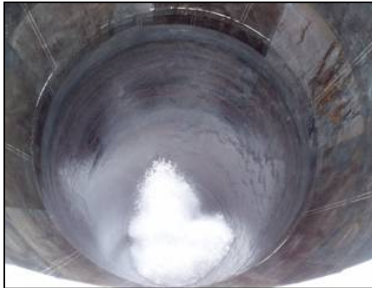
Figure 7. Liquid component of the Froth Zone formation as viewed from the top of the primary DynaWave ® inlet barrel during commissioning.
