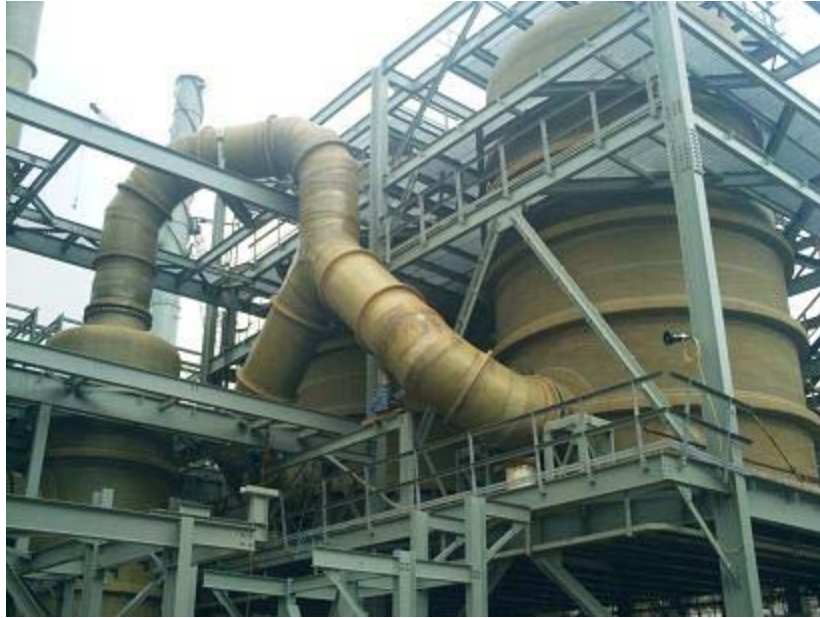
Figure 6. Dual wet gas mist eliminator vessels for a spent acid regeneration plant under construction.
